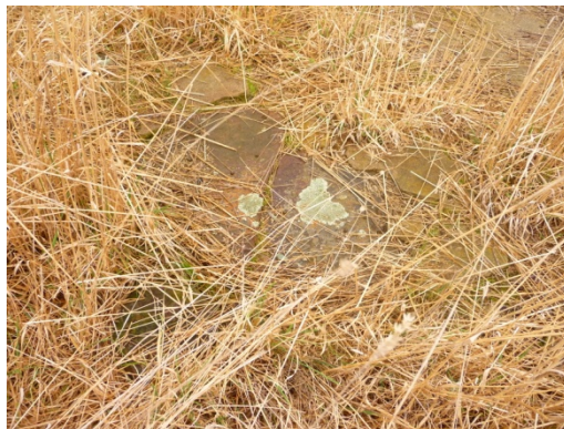
Foundation stones for what appears to be a second outbuilding near 1874 homestead
